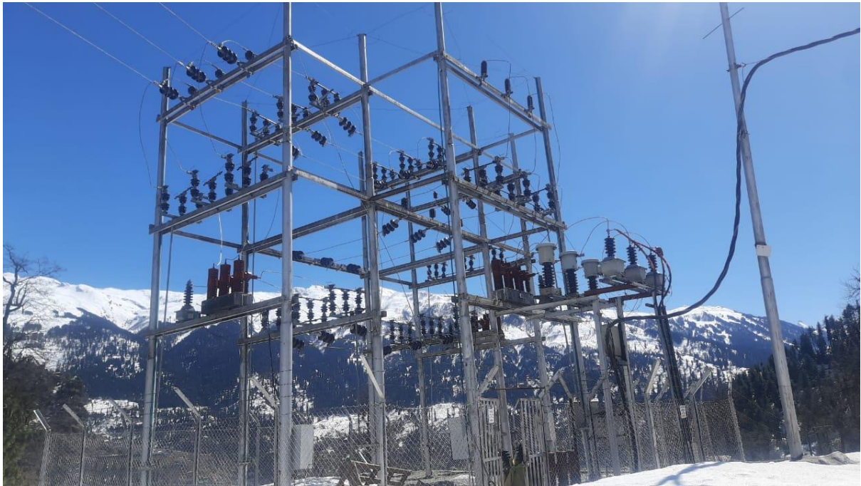
Figure-3: Electricity evacuation facility
